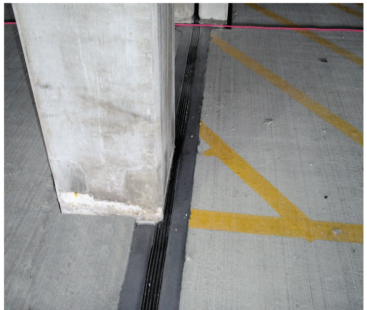
CR-400 Seal runs along side of column supports
