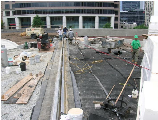
L.S. Decker crew installing expansion joints in plaza deck for the Phipps Towers
