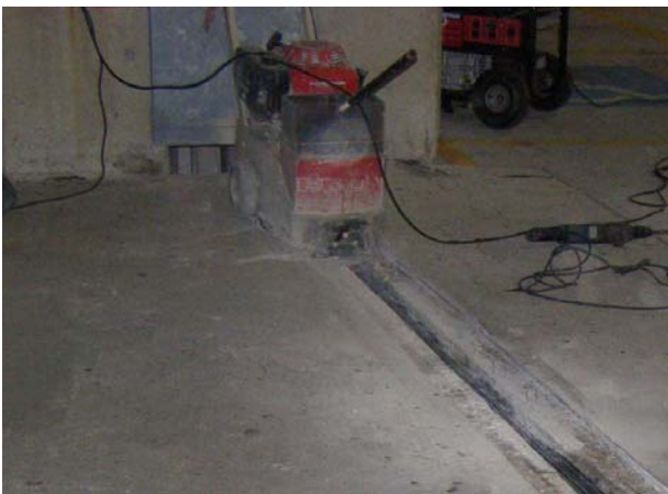
Twelve inch gas powered cup grinder used to remove contaminants and give a true and level surface from side to side as required for proper joint installation
