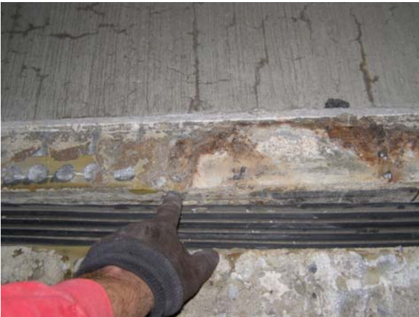
Existing blockouts needing extensive repair prior to installing new expansion joint
