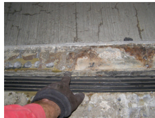
Existing blockouts needing extensive repair prior to installing new expansion joint
